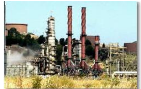
Distillation Columns at a refinery
