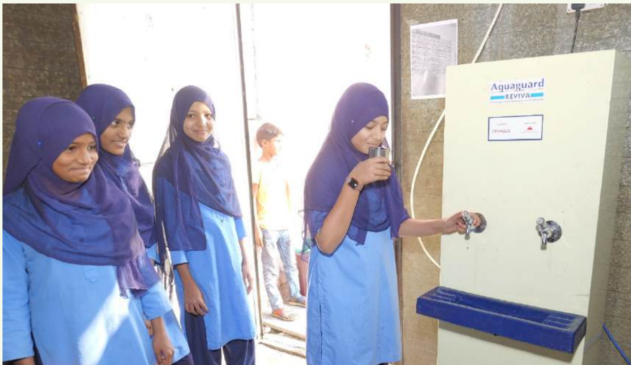
Girl students accessing safe drinking water from newly installed purification facilities under the Samarthanam project
