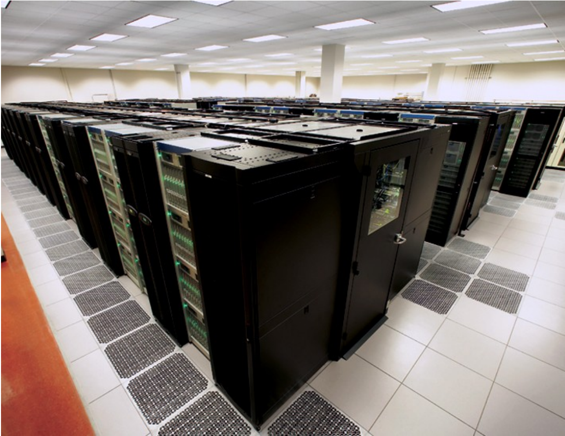
Figure 2-2. The Ranger cluster at the Texas Advanced Computing Center 3 .
